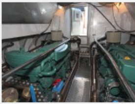
Seaward Nelson 35 Pilot Boat Engine Room
